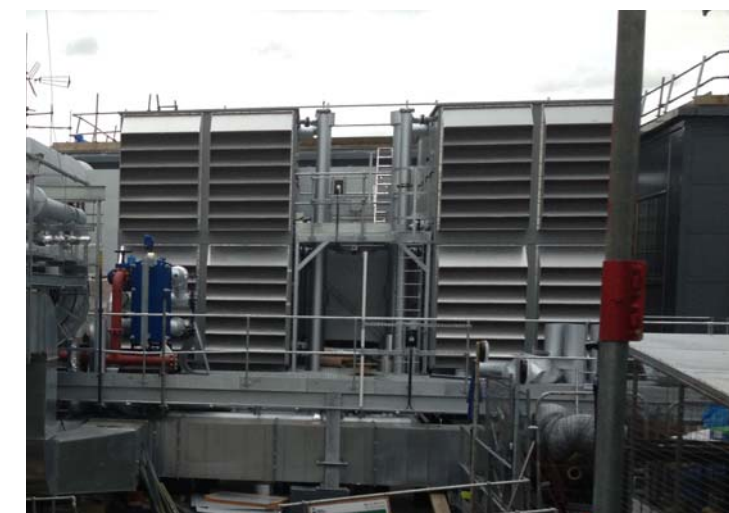
AHU X1 and X2 delivering 70M3\sec to central core of the building
