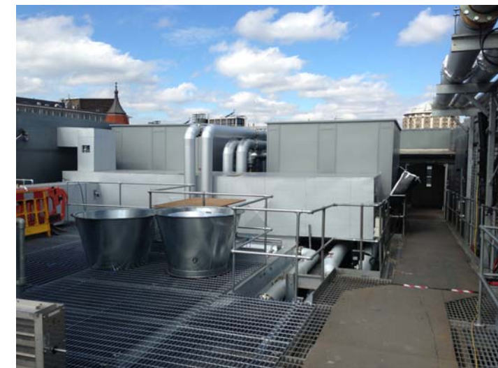
AHU S25 and S42 after refurbishment
