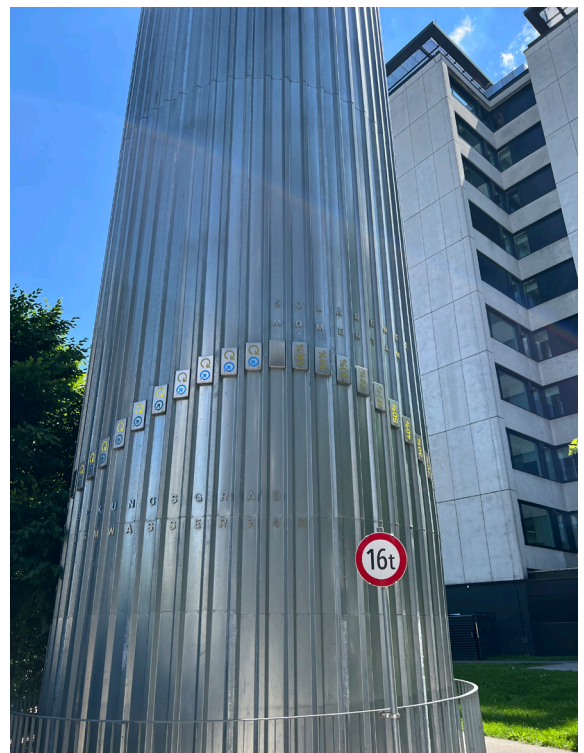
The buffer tank serving the whole development and connected to the heatpump running on exhaust air. The buffer tank features an interactive art work.
