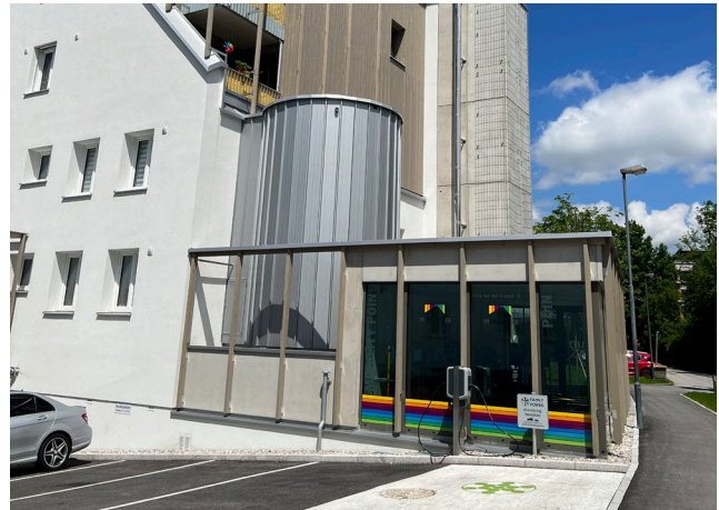
The buffer tank and the mobility point.
