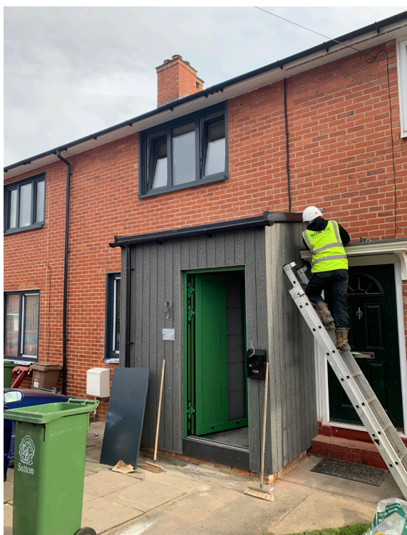
External 'porch pod' which houses the heating system and creates additional space.
