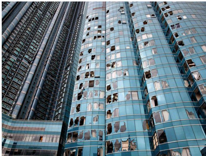
(Xinhua News Agency) Office building damaged after Typhoon Mangkhut
