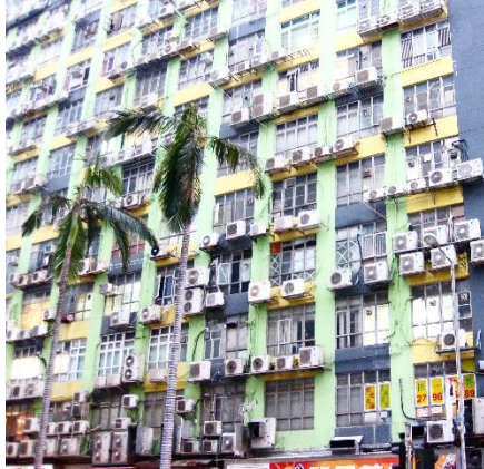
Typical heat rejection units arrangement in Hong Kong
