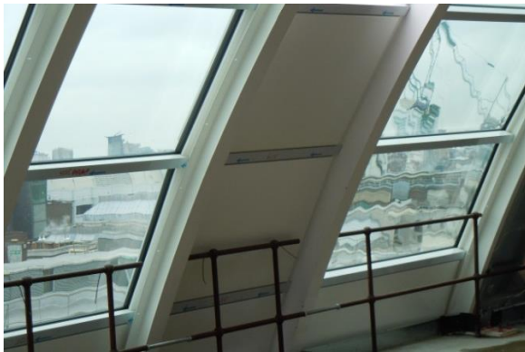
Figure 3.20: Anon project: Excessive roller wave in tempered cold bent glass.
