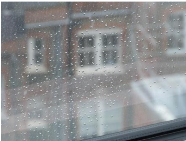
Figure 2.20: Bubbles in glass due to poor lamination. (Ramboll 2013)
