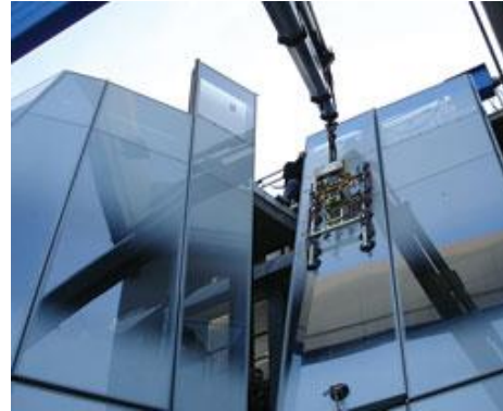
Figure 2.34: Installing the panels for the IAC Building New York, USA. (enr construction, 2015)
