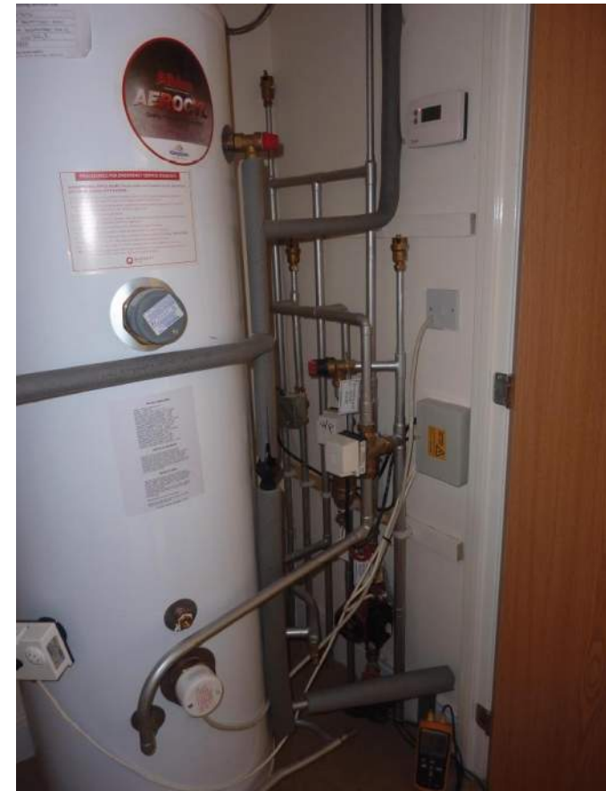
Hot water cylinder
