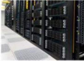
Data Centre and Mission Critical
